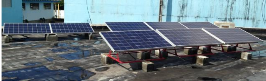
Figure 5 - Set of photovoltaic panels.
