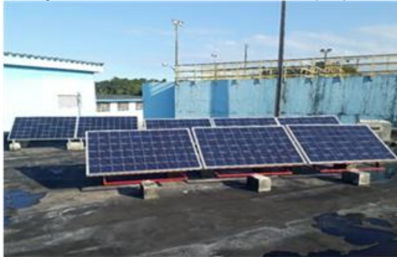
Figure 2.2 - Photovoltaic Modules from the BWD pilot plant
