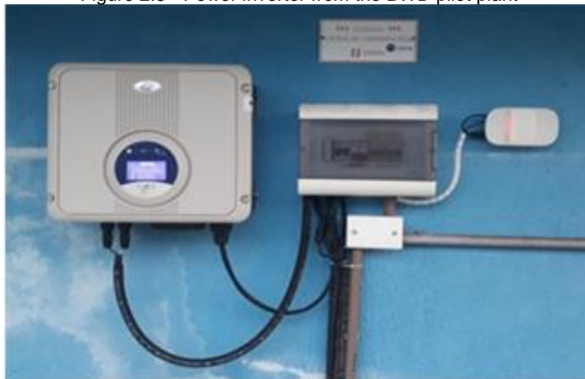
Figure 2.3 - Power inverter from the BWD pilot plant
