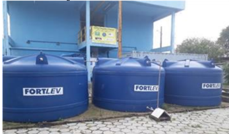
Figure 1.11 - Mixture water tanks
