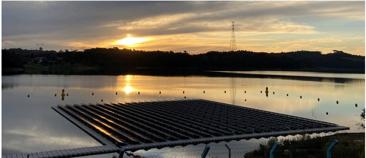
Figure 9 – Floating photovoltaic system at Passaúna reservoir
